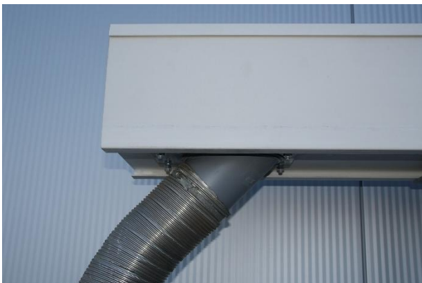
image 10, cable outlet flange
